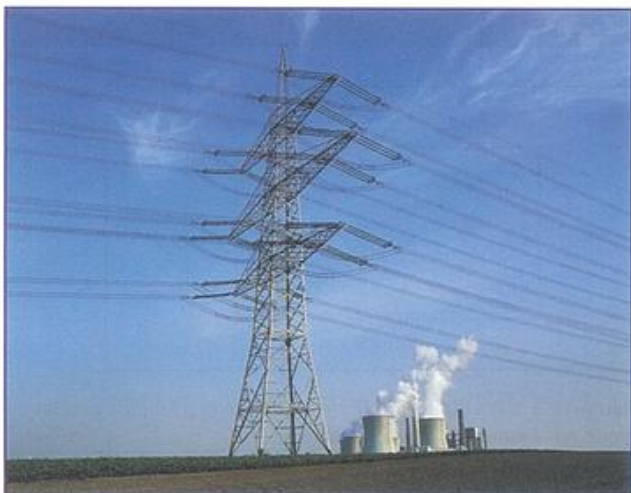
Figure 18.1 These cables carry large electric currents. Energy is being transferred from the power station to an industrial plant, where it will be used to turn machinery, split chemicals and so on.
