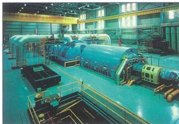
Figure 21.3 The turbine and generator in the generating hall of a Canadian nuclear power station. At the back are the turbines, fed by high-pressure steam in pipes. The generator is in the centre.
