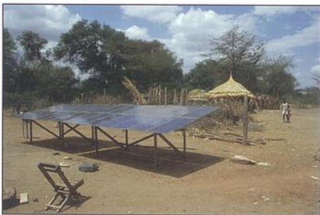
Figure 7.3 This array of solar cells provide electricity for a water pump in a Kenyan village.
