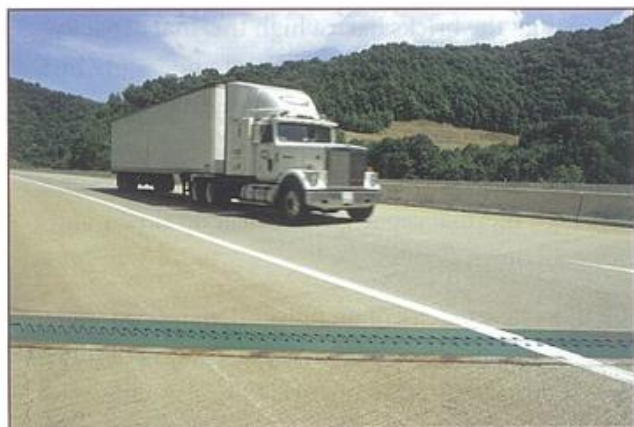
Figure 10.12 This truck is about to cross an expansion joint on a motorway bridge. On a hot day, the bridge expands and the interlocking 'teeth' of the joint move closer together.
