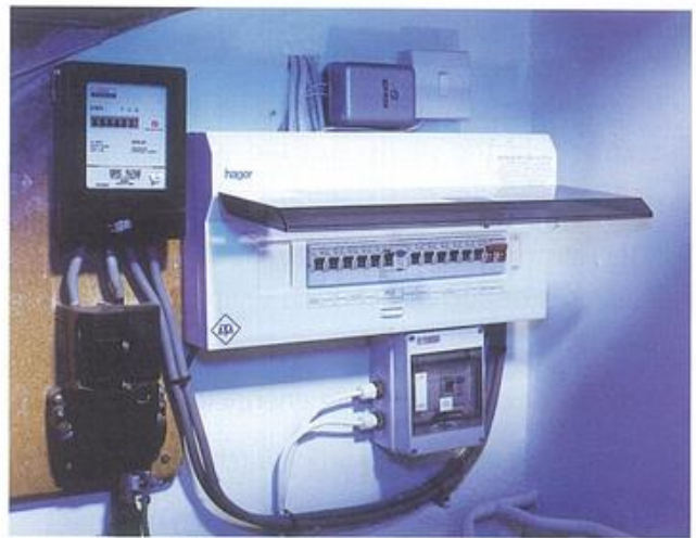
Figure 19.28 This is where the mains electricity supply enters a house. On the left is the meter. The white box contains a trip switch for each circuit in the house, together with an RCD, which protects the users of any circuit.
